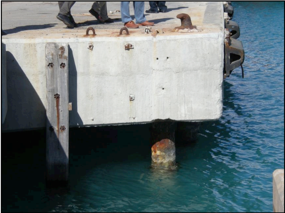
Figure F15 – Missing Ladder & Mooring Bollard Type 1
