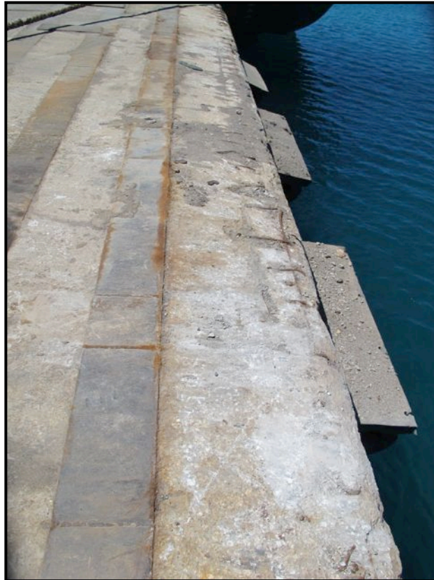
Figure F13 – Abrasion Damage to Main Jetty End
