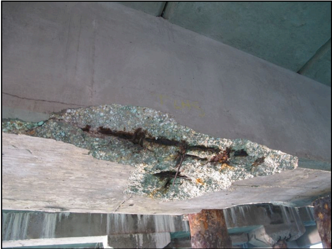
Figure F5 – Underside to Bent showing Spalling & corrosion to Rebar
