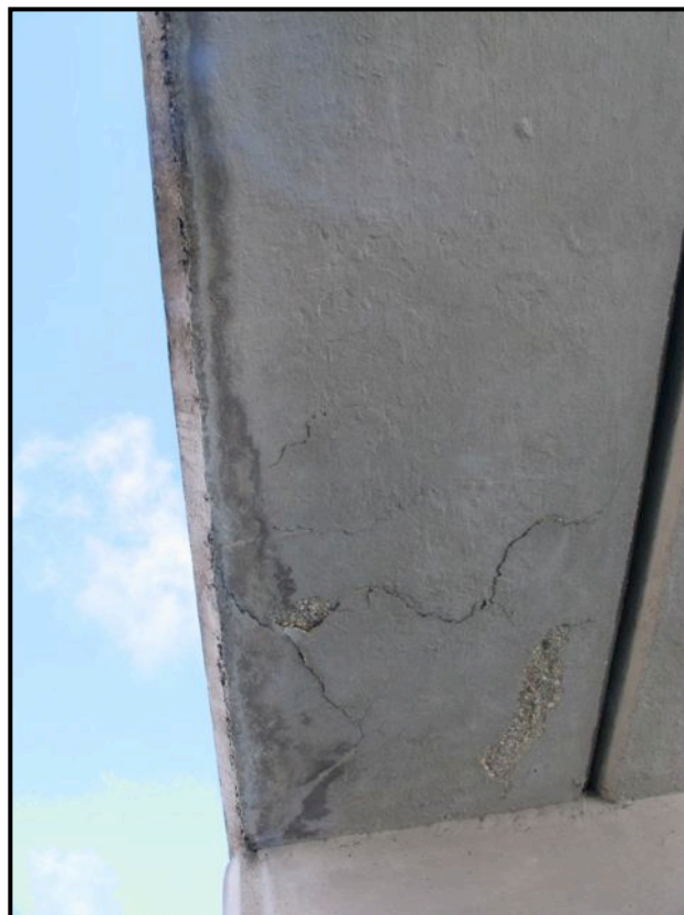
Figure F10 – Cracking to Main Jetty Approach Slab
