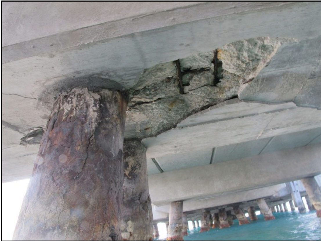
Figure F3 – Jetty Approach Bent Soffit Delamination & Corrosion of Raking Piles
