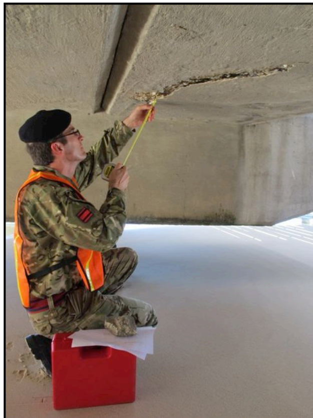
Figure F6 – Underside to Jetty Approach showing Slab Delamination
