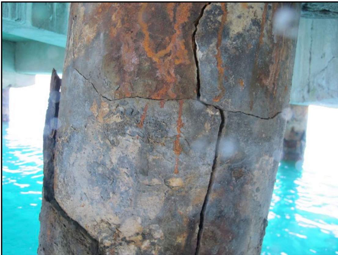
Figure F4 – Severe Damage to Failed Pile
