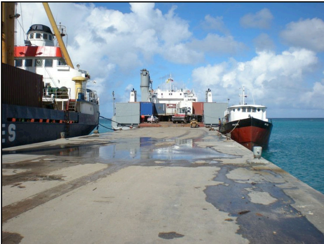
Figure F18 – Worn Surface of Jetty
