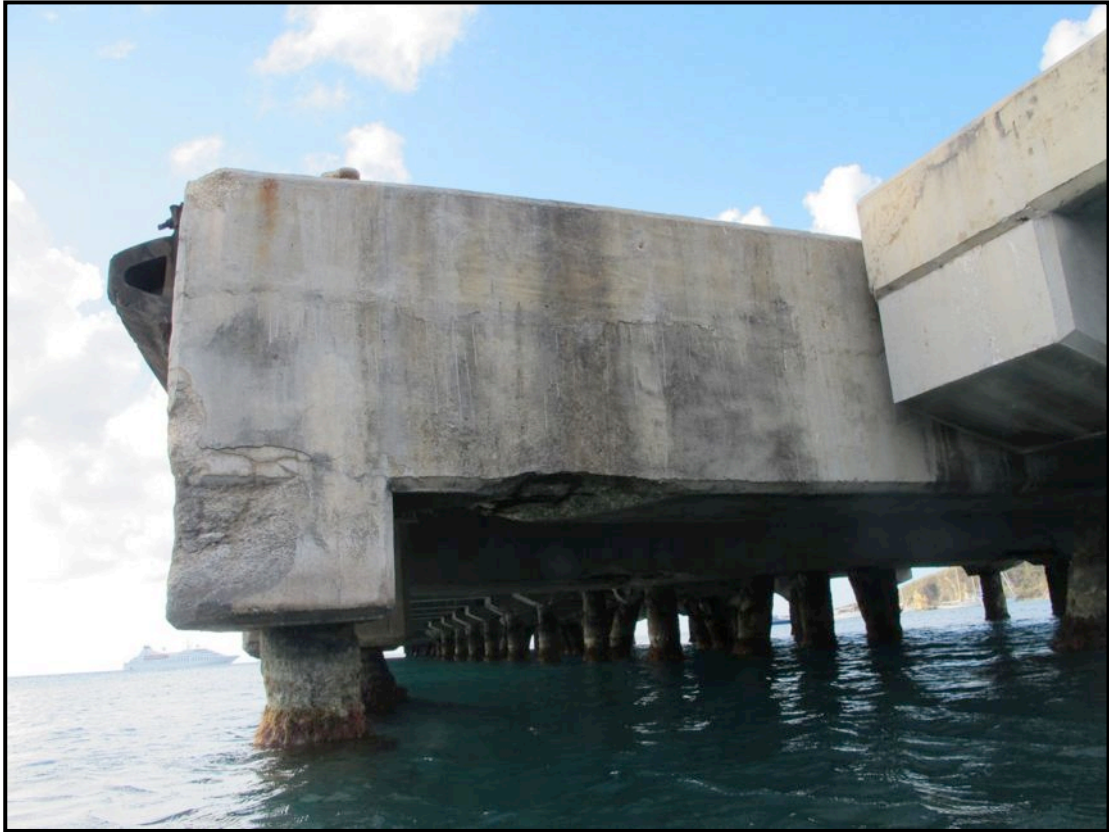
Figure F11 – Main Jetty Impact Damage
