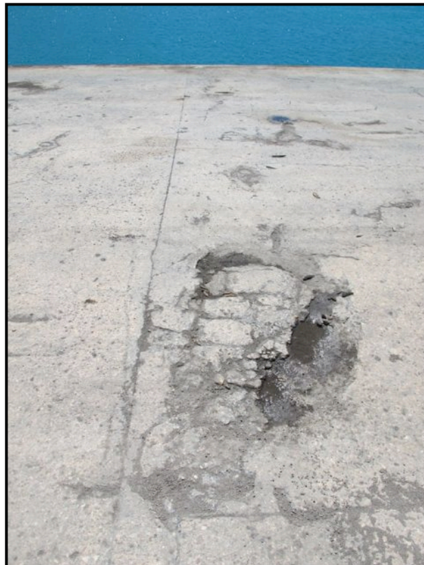
Figure F14 – Main Jetty Surface Degradation
