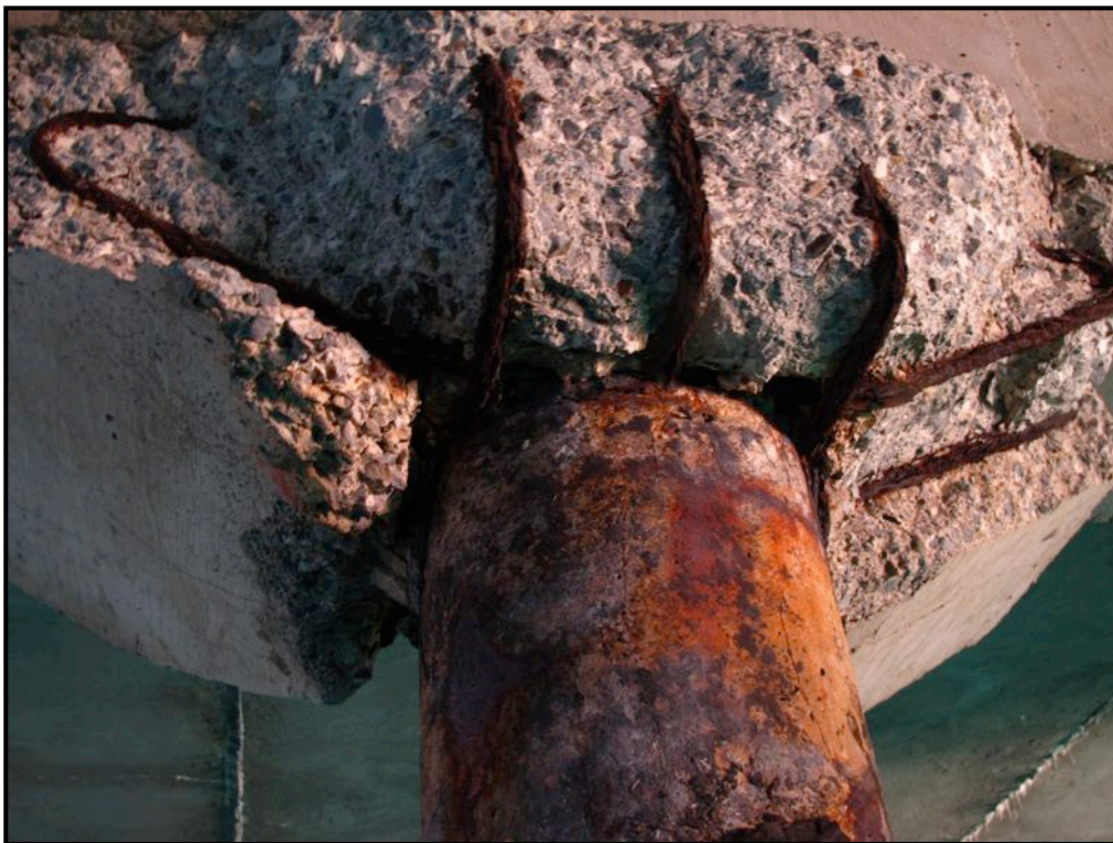
Figure F2 – Typical Pile Cap Corrosion
