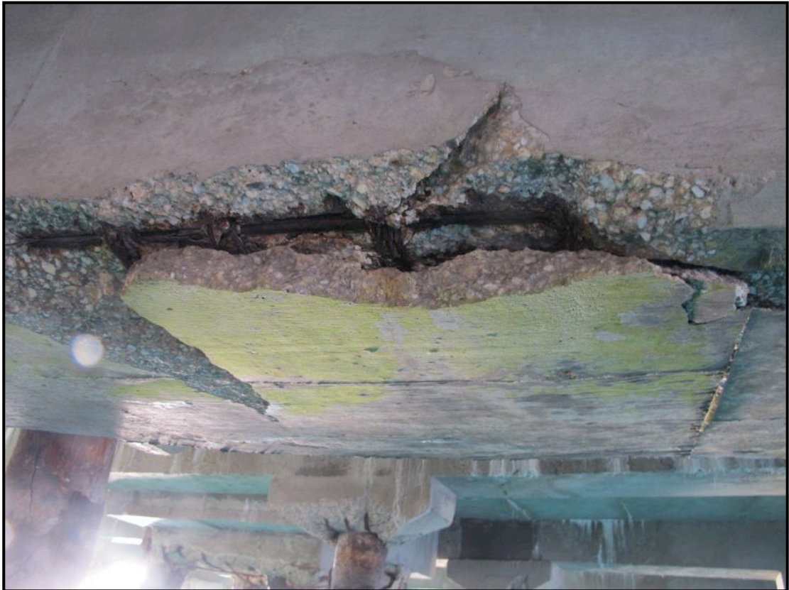
Figure F7 – Underside to Bent Showing Delamination and Rebar Corrosion
