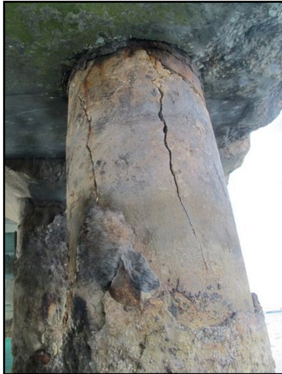
Figure F1 – Typical Damage to Pile
