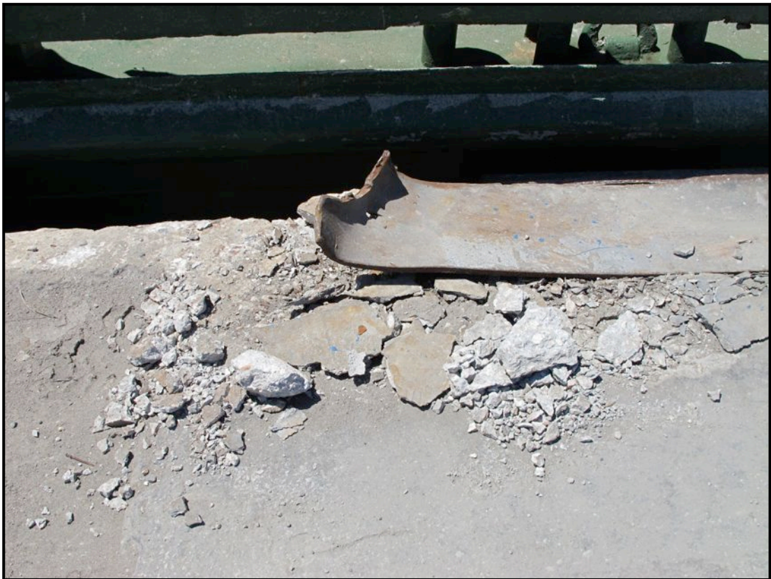
Figure F12 – Main Jetty Impact Damage to Edge Steel
